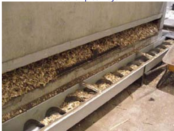
Wood Chip conveyor
