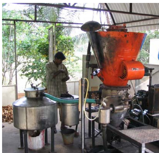
Figure 3. The 9 kW gasifier system installed for Odanthurai Panchayat water supply system in Tamil Nadu State.
